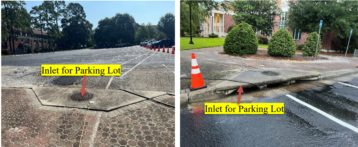
Figure 8. Inlet for Parking Lot from where Stormwater Runoff was Pumped by a Submersible Pump to Field Test Site
