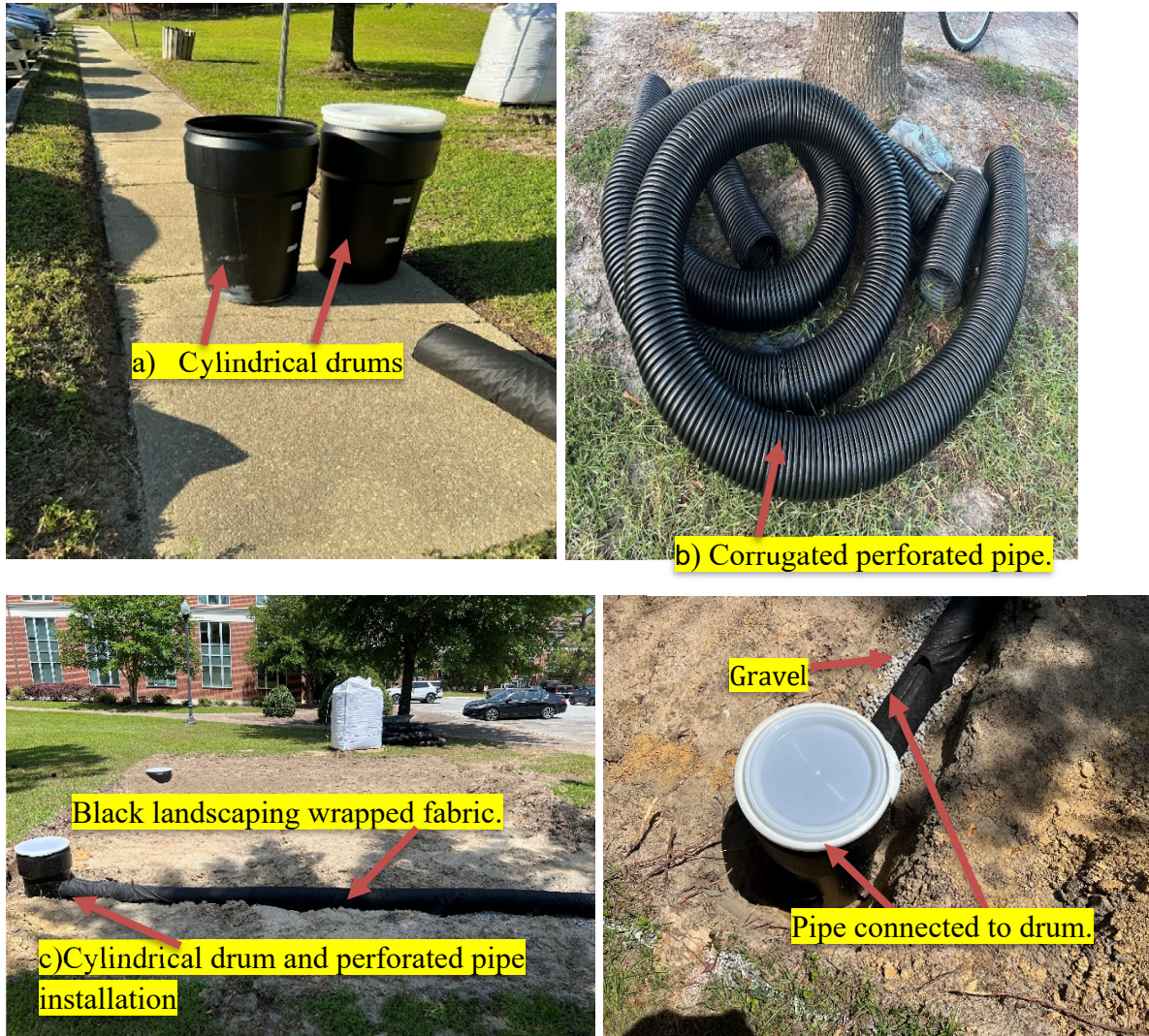
Figure 15. a) Two cylindrical drums b) Corrugated perforated pipe c) Cylindrical drum and perforated pipe installation
