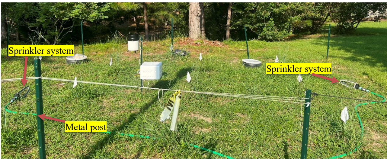
Figure 19. 1/3-HP 115-Volt Submersible Utility Pump with sprinkler system
