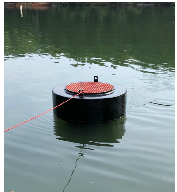
Figure 4. Impoundment outlet device that collects and discharges cooler, mid-depth lake water.
