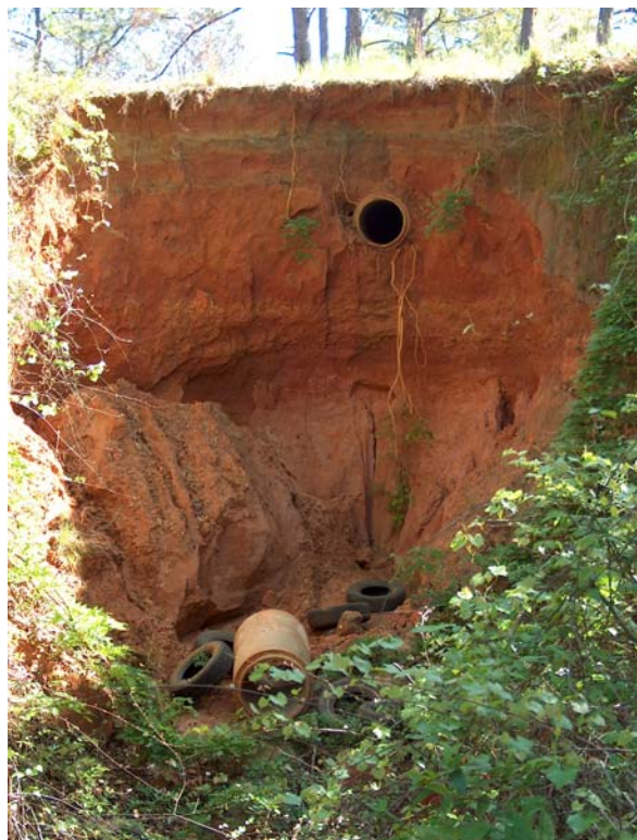
Figure 6. Rapid and significant erosion at south end of culvert across county road in Fig. 5. Note four-foot segment of culvert that has broken off and tires for scale. Another segment lies beneath large block of sediment just behind visible section of culvert.
