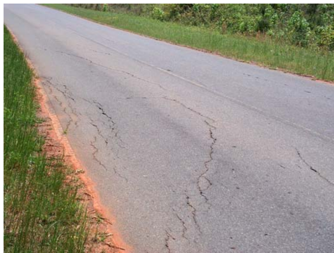
Figure 8. Concentric cracks signifying initial road failure are centered over a culvert at the head of an erosion gully.
