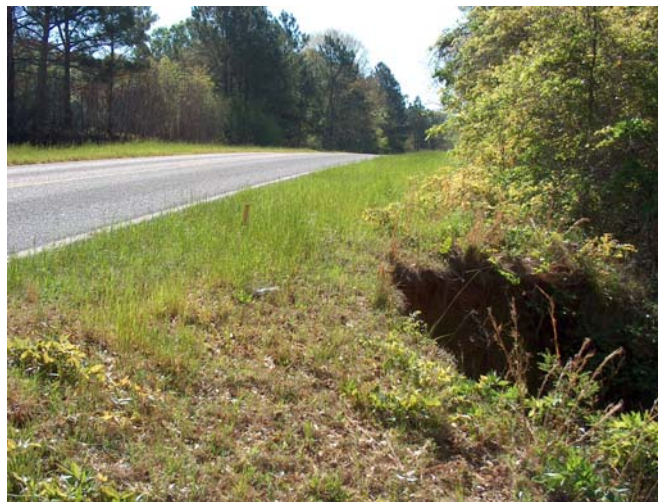
Figure-7 Top of gully shown in Fig. 6 lies within six feet of county road.
