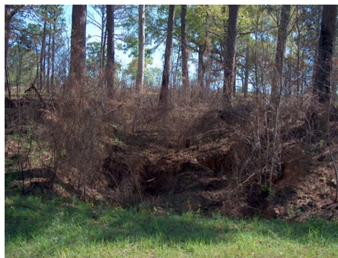
Figure-5 Drainage above culvert pictured in Fig. 6 Entrance to north end of culvert is just above grassy area in this picture.
