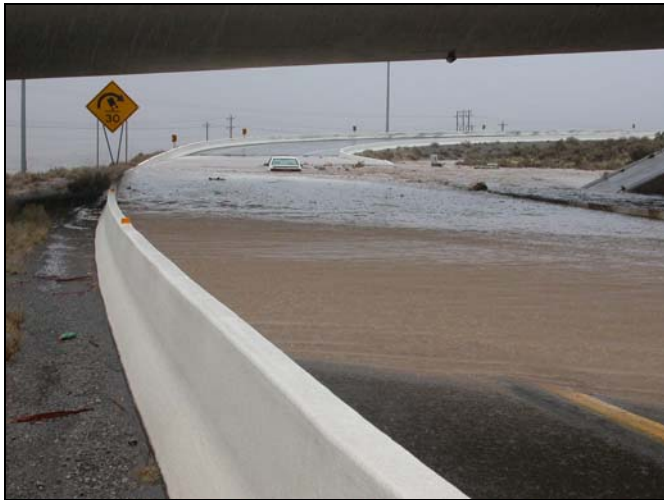
Figure 1. Flooding of SR395 on-ramp (12/31/05)
