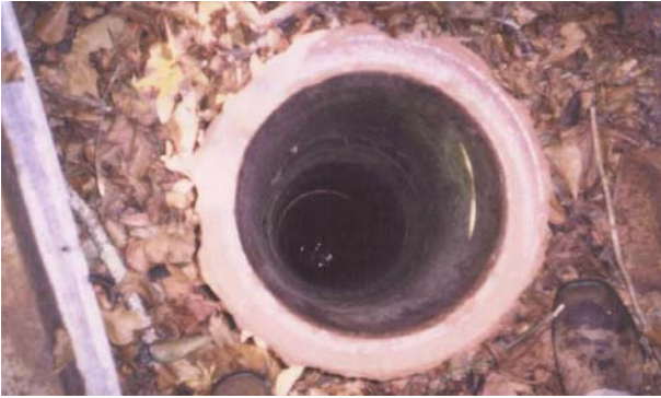
Figure 3. Abandoned 12-inch bored well with terracotta casing that had deteriorated and posed
